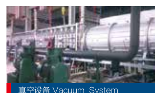
真空设备 Vacuum System
