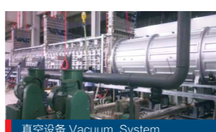
真空设备 Vacuum System
